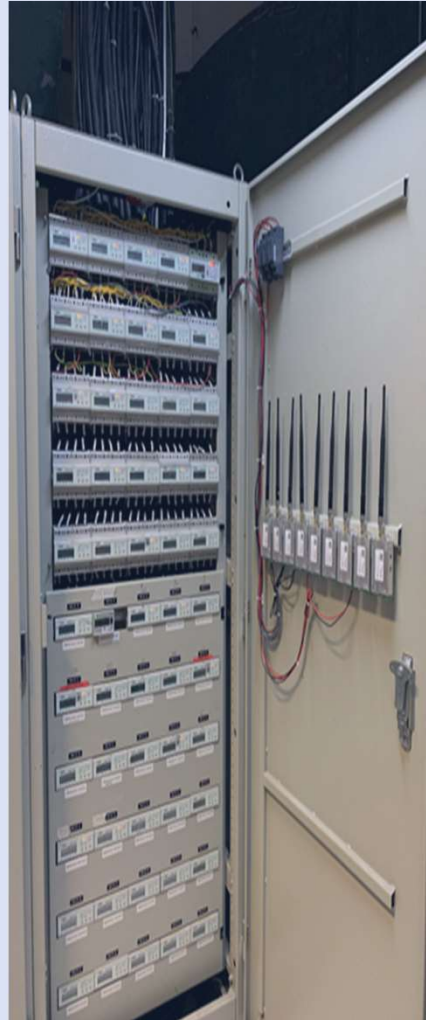
RTU FOR ENERGY METERS
